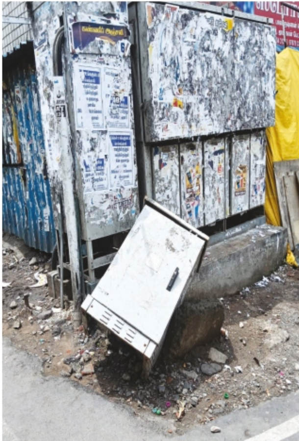
BREAKDOWN BOX : This internet cable box a hindrance to pedestrians and motorists at SM Blocks Sathyamurthy Street, Jafferkanpet. Will concern officials remove for the safety of public.
